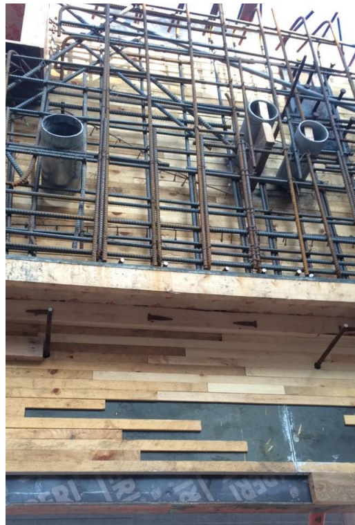
Figure 31: Pre-fabricated wooden Board form placed inside steel concrete form with rebar being set.
