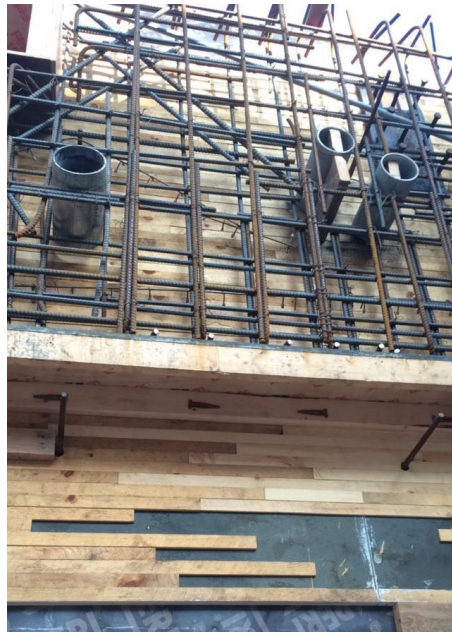
Figure 38: Board formed concrete lining inside Peri Trio form with rebar cages and dowel insertion connectors.
