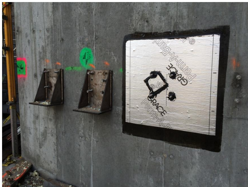
Figure 1: Bracket-anchor system to support Lecce Limestone Panels & waterproofing barrier on DRUM Façade
