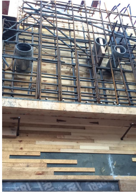
Figure 4: Pre-fabricated wooden Board form placed inside steel concrete form with rebar being set.
