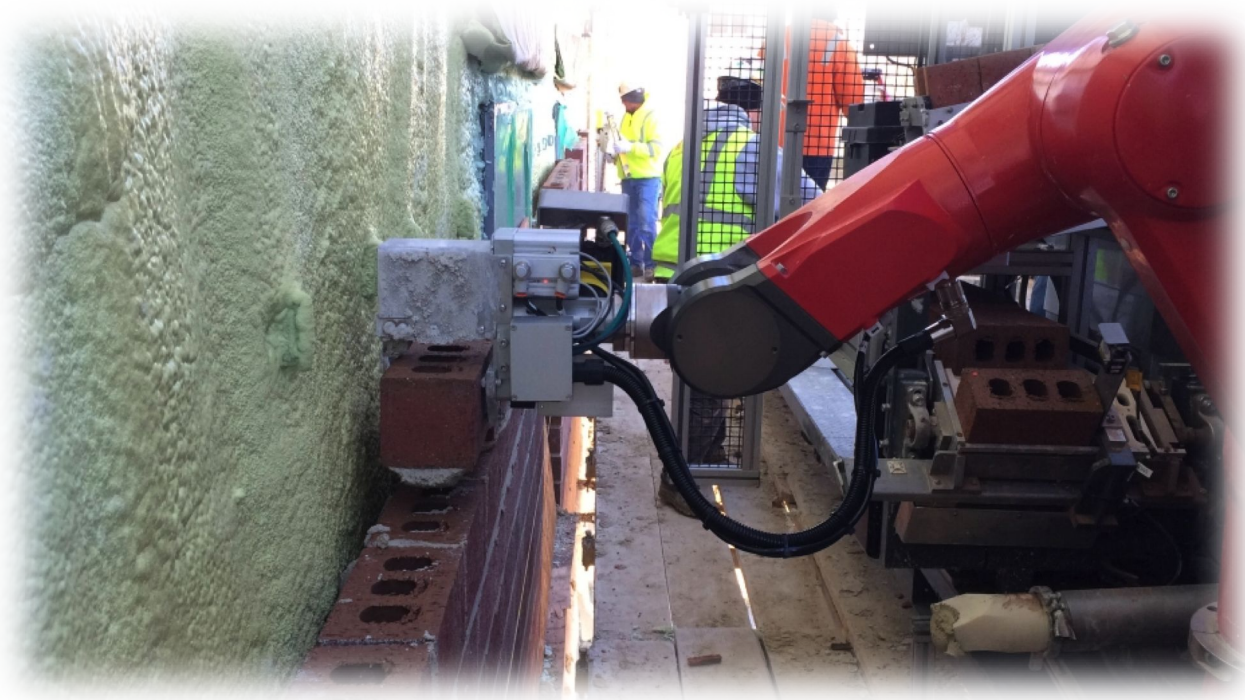
Figure 1: Semi - Automated Mason laying brick at Fort Lee Barracks Job in Virginia
